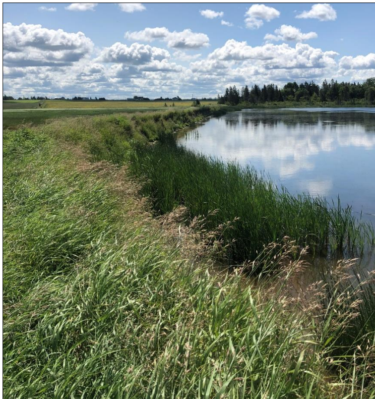
Photo 3. Significant erosion on Amherst Point 1 outer dyke (northeast dyke).
