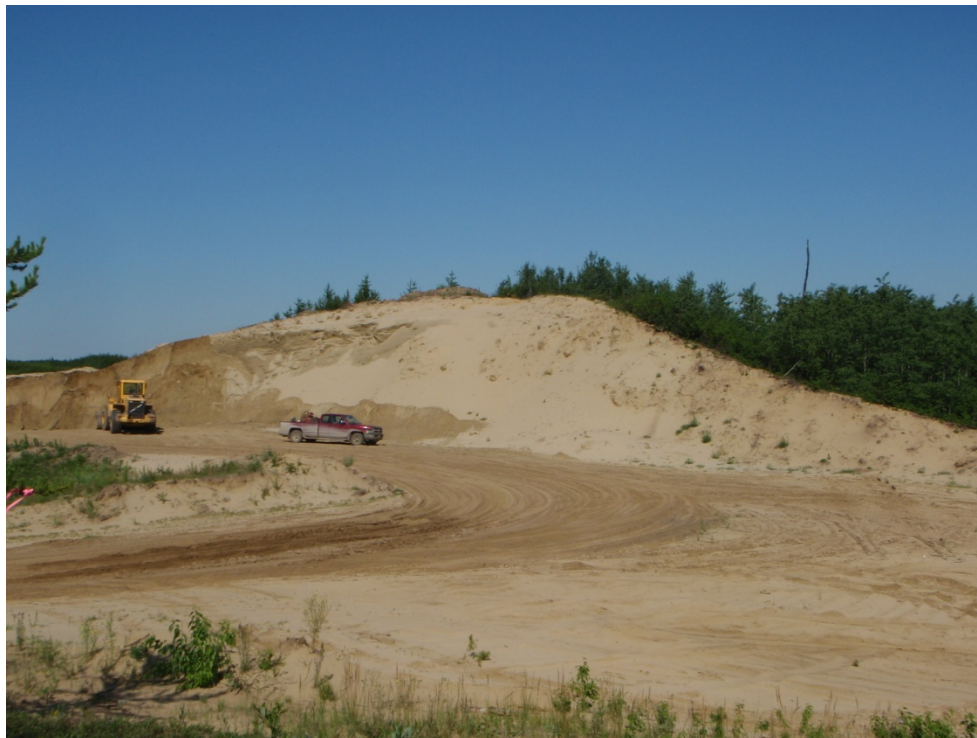
Photo 45: View looking west toward excavated ridge where part of FhNe 57 is located
